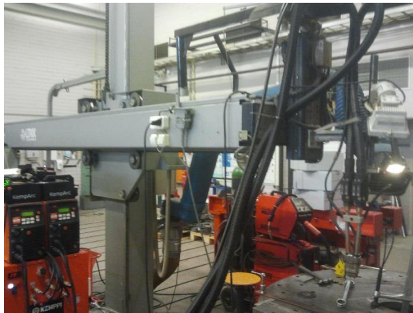
Figure 22. Power sources, cooling unit, welding column and torch.
