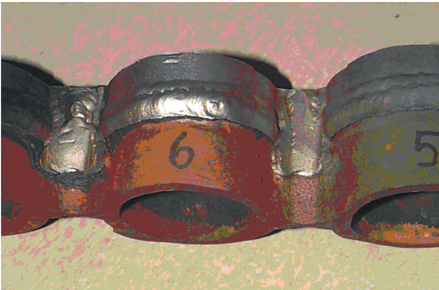
Figure 10-15, Galvanic corrosion of carbon steel.
