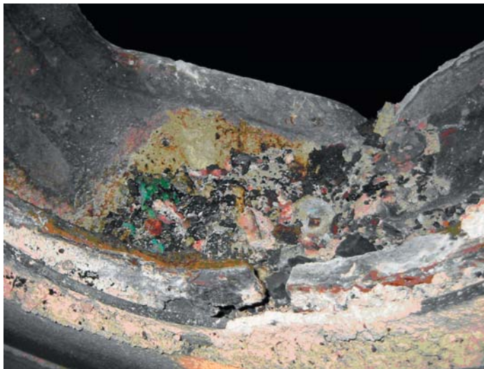
Figure 10-17, Corroded load burner sleeve.
