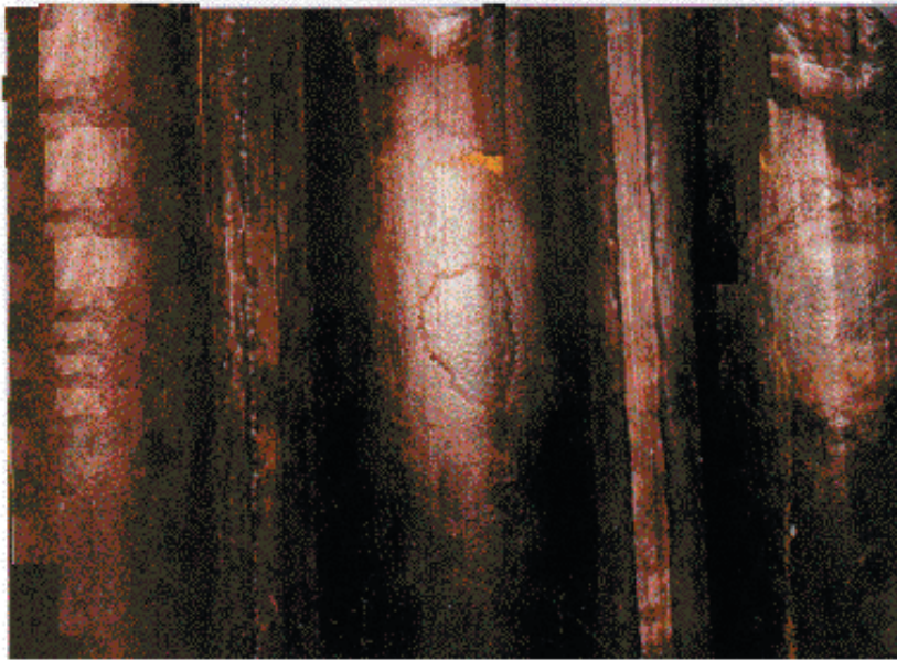
Figure 10-13, Cracked 304L floor.
