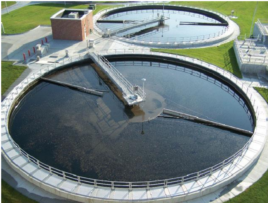
Picture 10: A circular sedimentation tank (City of Lincoln)
