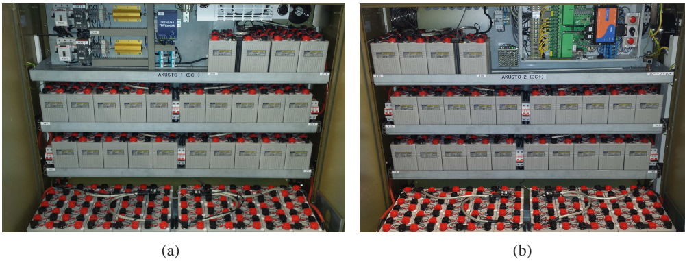
Figure 6.5: Back-to-back installed A and B cabinets with pull-out battery shelves. The main circuit control components are installed in cabinet A (a) and the control electronics in cabinet B (b) (Publication IV).
