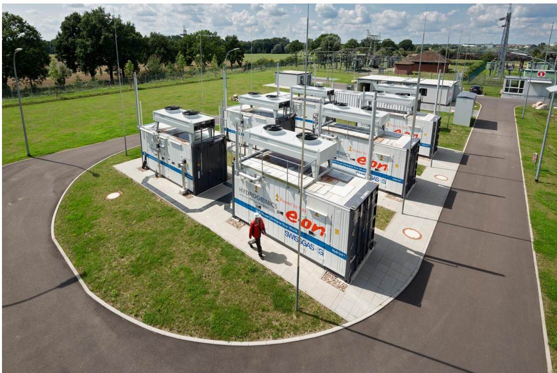
Figure 17: The WindGas plant in Falkenhagen [81].
