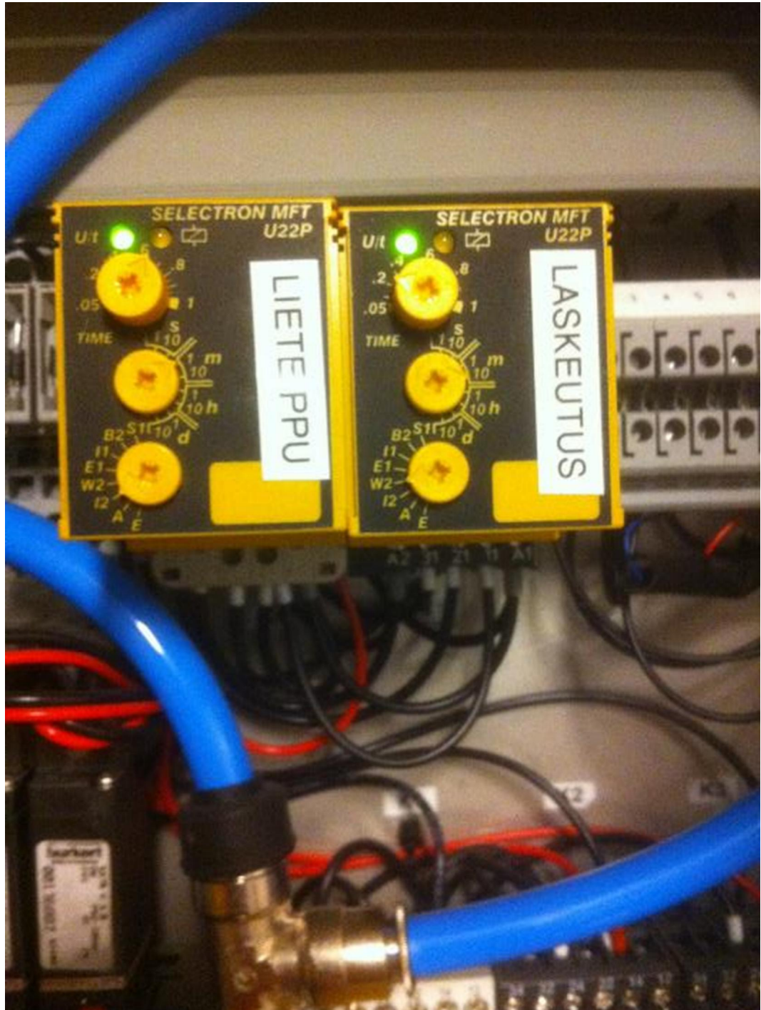
Figure 7. Relay units for slurry pump and settling tank and set times to control.
