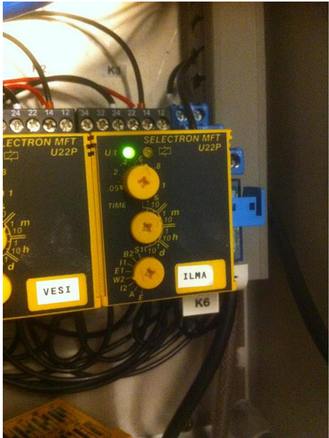
Figure 16. Time relay for air feed valve ILMA and time setup for the control.
