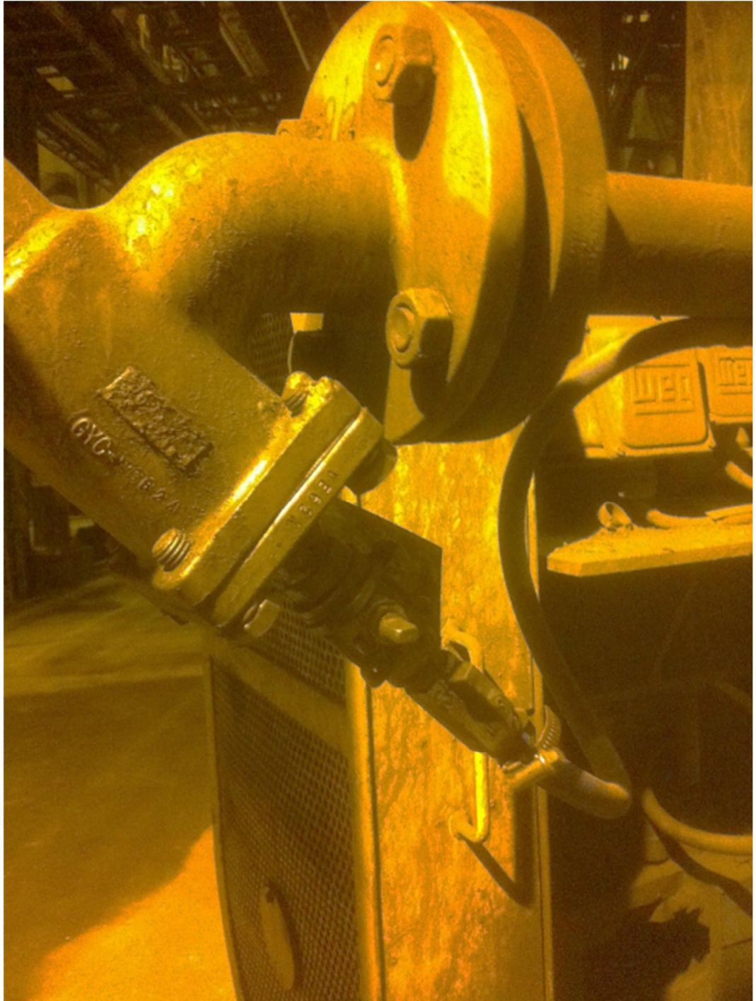
Figure 18. Sample point for the process water is through the valve seen in bottom of the connector.
