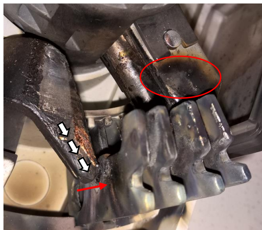
Figure 3.26 White arrows pointing the arc movement during contact breaking. Red arrow pointing damage of arcing plate due to arc picking and the same effect is encircled by a red circle.
