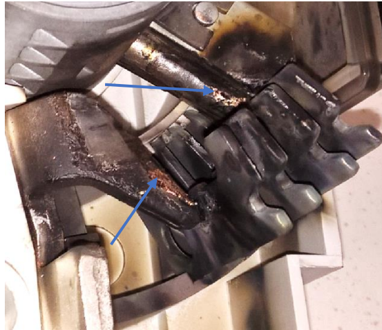
Figure 3.25 Blue arrow heads are showing points on the contacts where contacts are melted due to arc generation.
