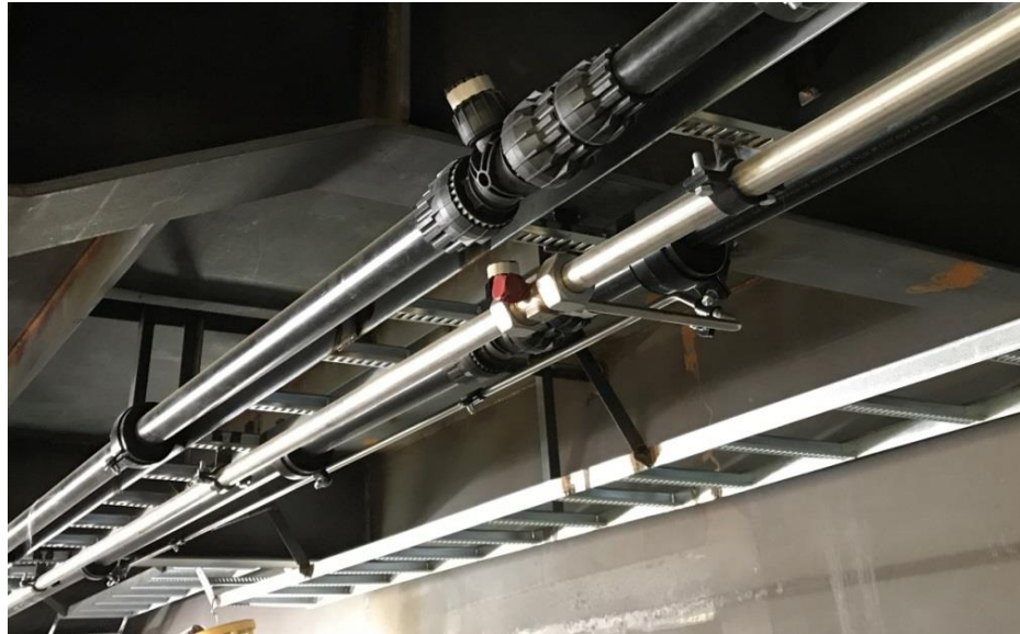
Figure 26. Corridor piping module
