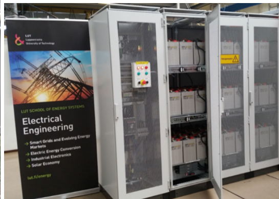
Figure 55: Green Campus (GC) BESS.
