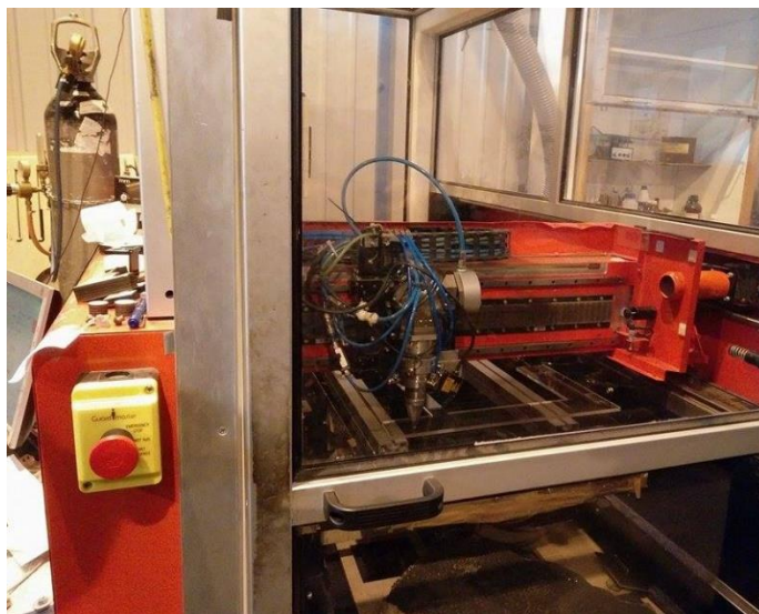
Figure 27. CO 2 laser workplace, protecting housing.
