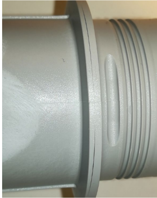
Figure 21. An example of cracking in the PPSU fittings flange in chemical testing.
