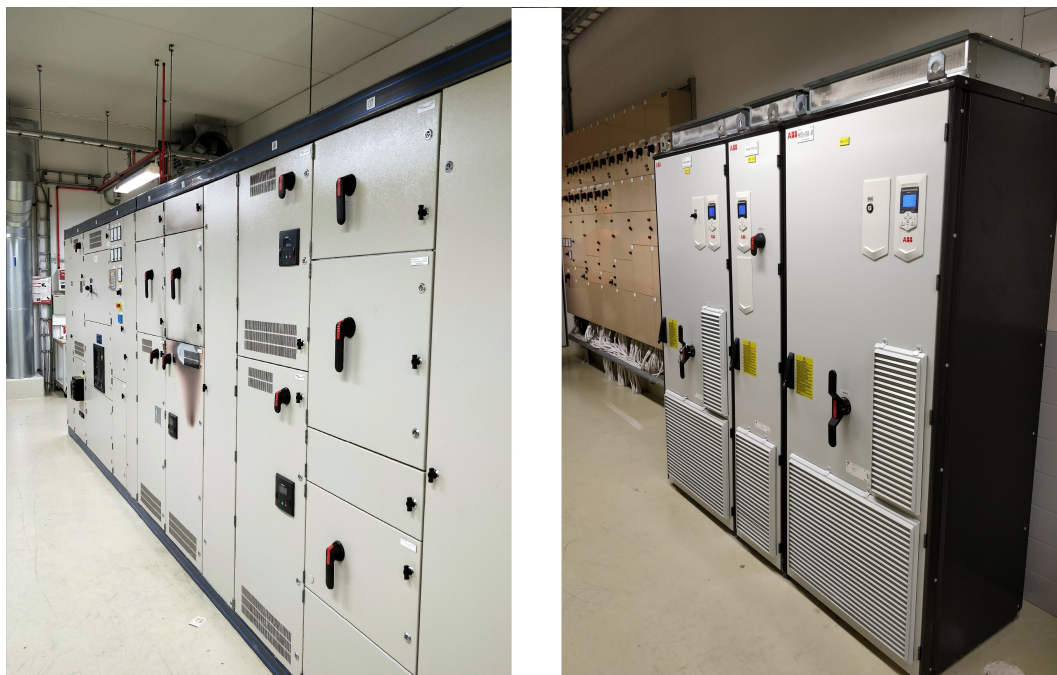
Figure 4.4: Small frequency converters are installed in hubs as shown on the left. Bigger ones have their own cabinets like the ones on the right.
