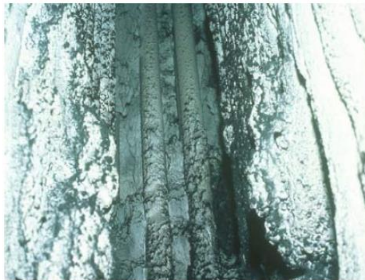
Figure 13. Massive deposit on boiler bank tubing. (Honghi Tran 2015, p. 7)
