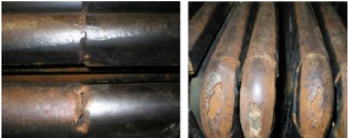
Figure 17. Examples of erosion damage on boiler tubes (Wojnar 2013, 475).
