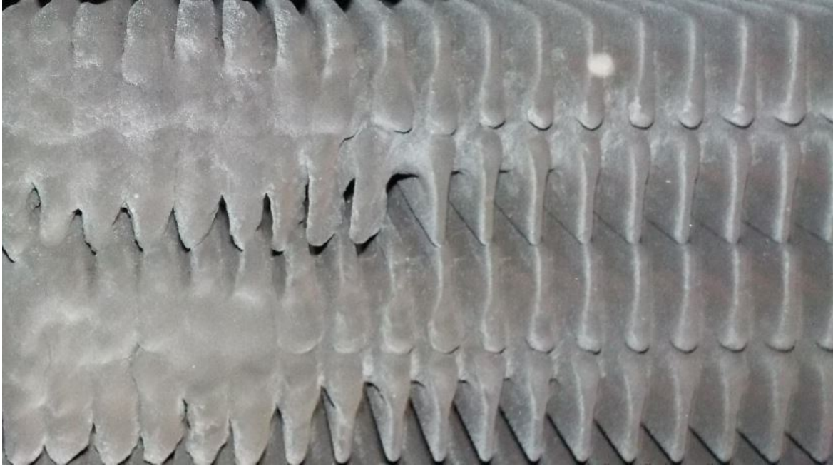
Figure 28. An almost clogged tube bundle in a WHRB after a reciprocating engine burning LBF. The WHRB was running for an extended period with a broken rake soot blower which was left unnoticed.
