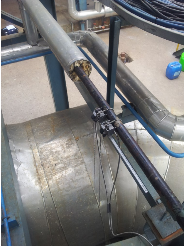
Figure 25. Fluxus measurement head clamped to feed water piping which have its insulation removed from measured section, with direction of water flow being toward the photographer.
