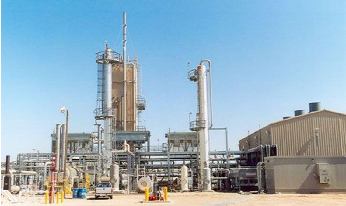
Figure 3.10: Crude Helium Enrichment Unit (BLM, USA).
