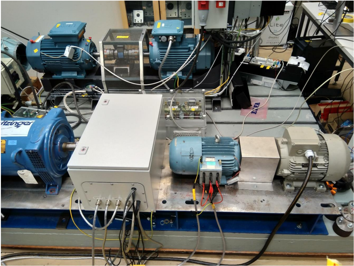
Figure 5.1 The testbed and electrical machines used in the study. The brown asynchronous machine is used to emulate the synchronous machine rotor. Light blue machine is the slip ring asynchronous machine used as an asynchronous exciter. The grey box between blue synchronous machine and SR machine contains the diode bridge, clamps and current transformers used in this study. In the left side is the blue synchronous machine, the stator side is open circuit.
