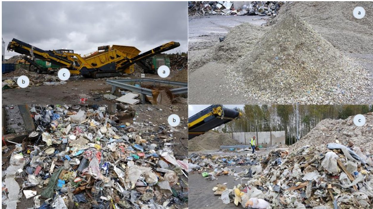
Figure 4. Mobile Keestrack screen separating crushed mixed C&D waste: a = fine underflow, b = magnetic fraction, c = energy waste with other material continuing to air classifier. © Havukainen.
