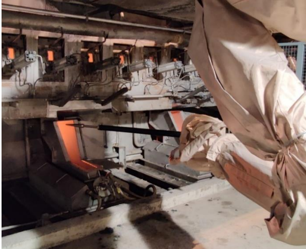
Figure 23. A commissioning of the hood cleaning program can be time-consuming for the middle smelt spout due to the limits of the robot's axes and the location of the smelt spout.
