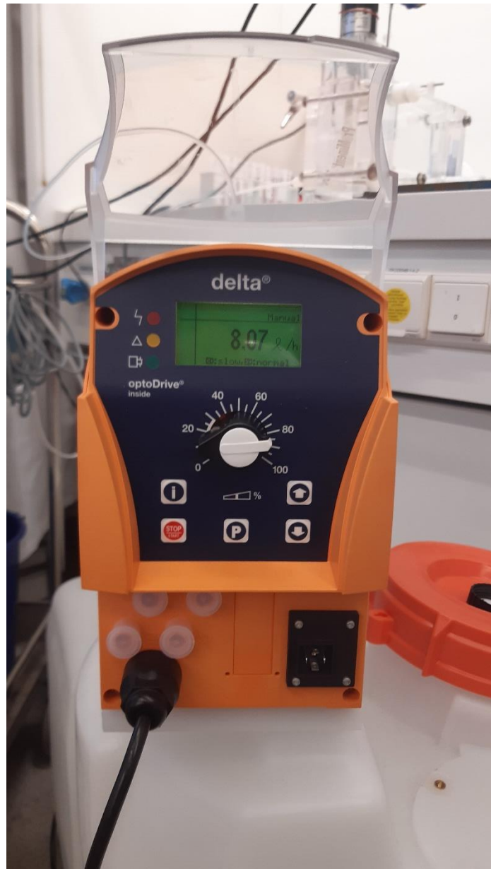
Figure 22. Diaphragm pump used to feed deionized water to the mixer
