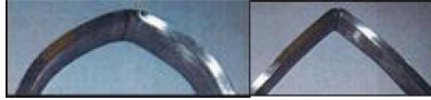
FIG. 9. The bent profile of the weld, left: undermatching filler, right: matching filler material.
