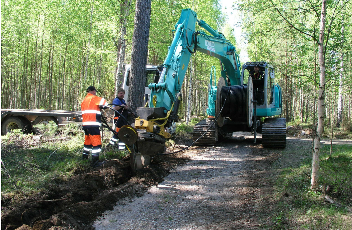
Picture 2.6 The process of ploughing the 1 kV cable [Photo by Pasi Kaskinen, Source: 5]
