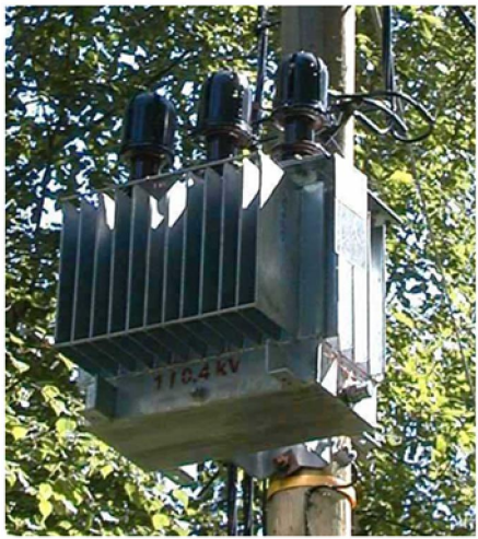
Picture 2.9 1/0.4 distribution transformer [5]
