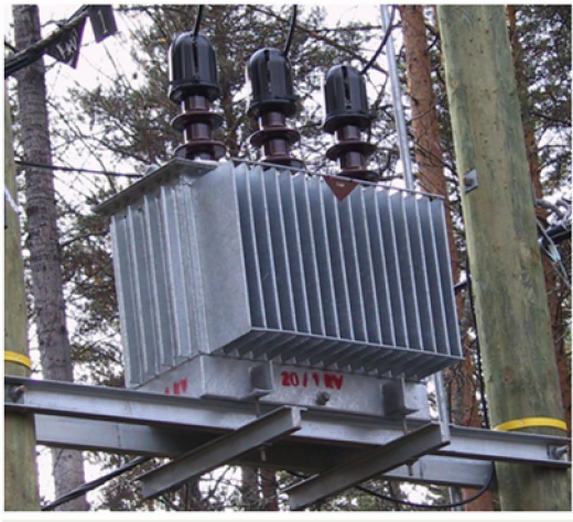
Picture 2.7 20/1 kV distribution transformer [5]
