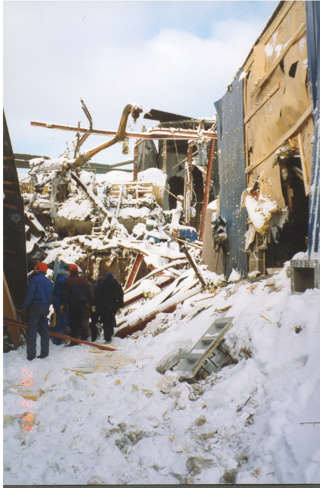
Fig 5.14. View from the same direction as in Fig. 5.13. The people give the scale [31].
