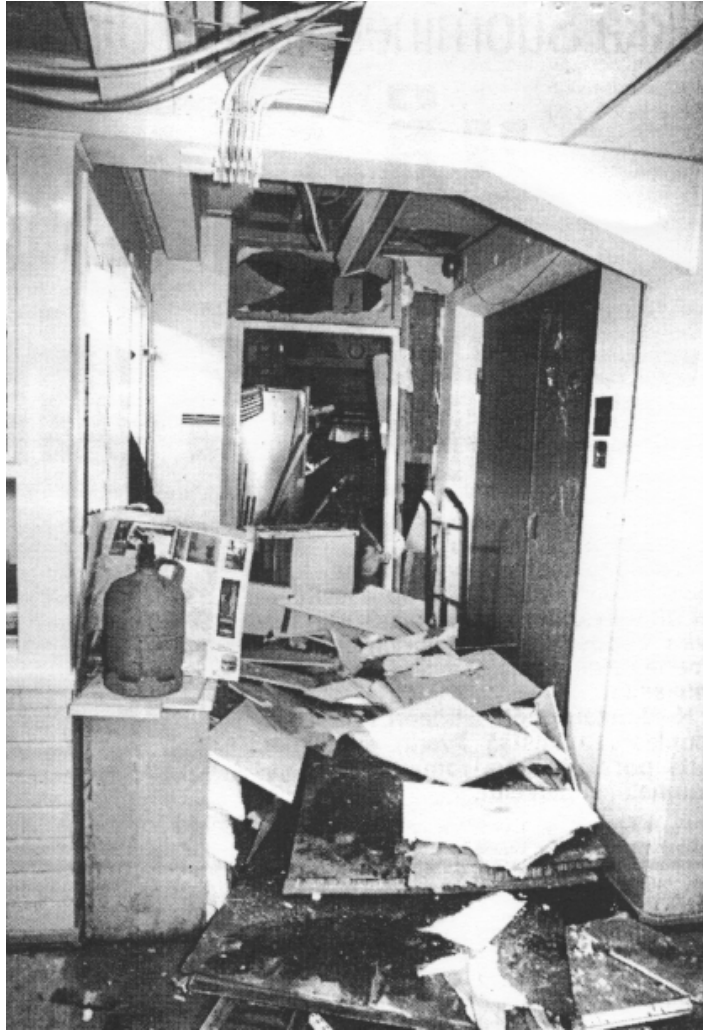
Fig. 5.10. The lobby of the laboratory after the explosion of a steam generator, which occurred in the room in the back. The isentropic exergy was about 6 MJ [30].
