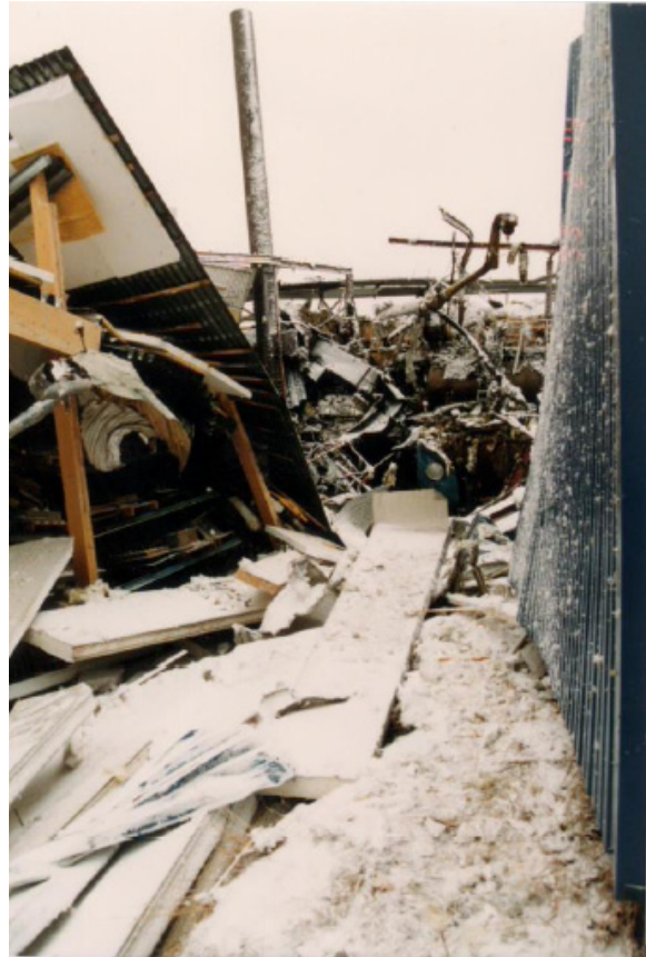
Fig. 5.13. View from the south direction [31]. The destroyed boiler house with the declined chimney is on the background. The collapsed storage wing is on the left.
