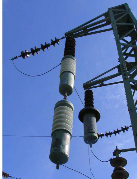
Fig. 1.1: Coupling capacitors in the HV distribution network.
