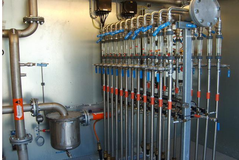
Figure 19: LFG treatment, conditioning and analyzer
