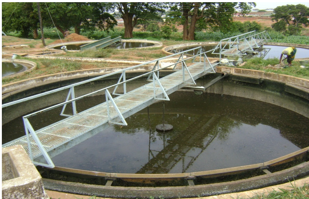
Fig. 2.6 Humus tanks at Soche WWTW, similar to Blantyre WWTW
