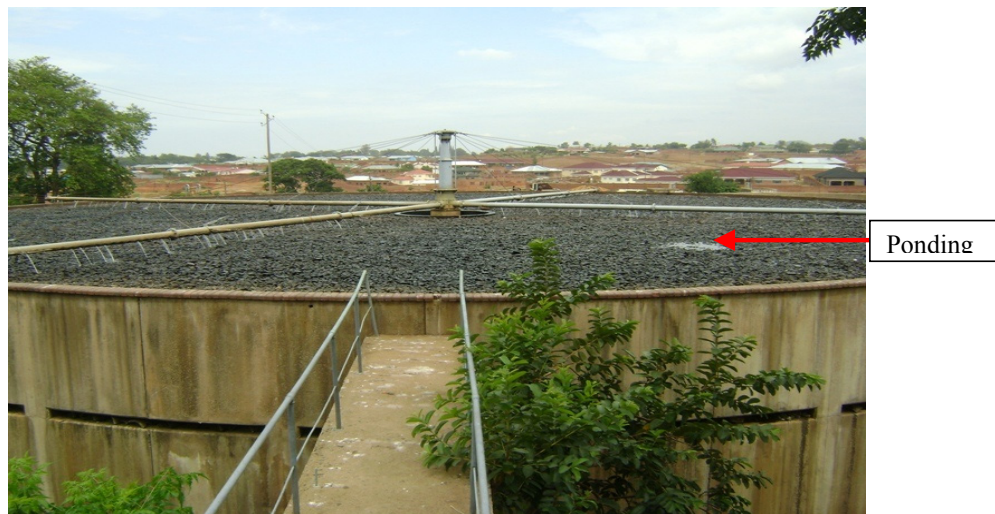
Fig. 2.5 Trickling filters at Soche WWTW, similar to Blantyre WWTW
