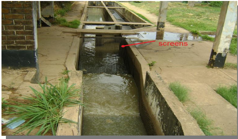
Fig. 2.4 Bar screens are followed by parallel constant velocity grit chambers at Soche WWTW. A similar set up is available at Blantyre WWTW
