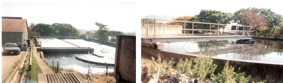
Fig. 2.12 Treatment units at MDW&S with oxidation ditch (L) and sedimentation tank (R) situated downstream of oxidation ditch
