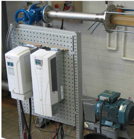
Fig. 1.4: Frequency converters of the laboratory setup used in this study. Modern frequency converters include several pump-related monitoring and control functions, such as the sensorless calculation of the pump flow rate.
