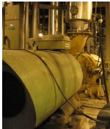
Fig. 3.19: Pulp pumping system in a paper mill. The pulp pump is located next to the paper machine 3, and it transfers the fluid from a reservoir to the tanks near the paper machine.
