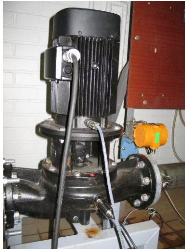
Fig. 4.37: Grundfos pumping system. It consists of a Grundfos LP 100-125/130 centrifugal pump and a Grundfos induction motor. The rotational speed of the pumping system was controlled with an ABB ACS 800 frequency converter.
