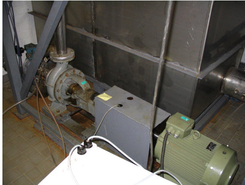
Fig. 4.33: Serlachius pumping system. It consists of a Serlachius DC-80/260 centrifugal pump and a Strömberg induction motor. The rotational speed of the pumping system was controlled with an ABB ACS 800 frequency converter.
