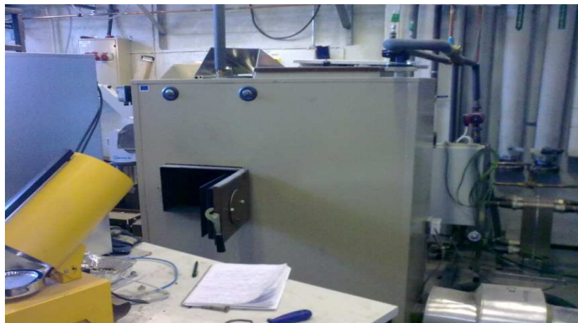
Picture 17. Side picture of VETO boiler at Energy laboratory of LUT /50/.
