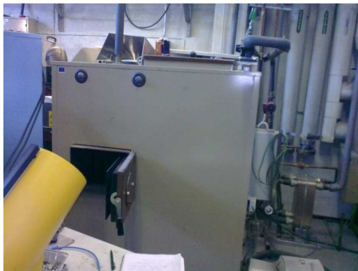
Picture 16. VETO grate boiler at Energy laboratory of LUT /49/.
