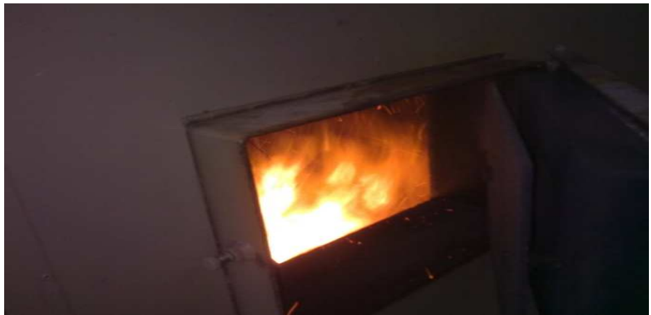
Picture 26. Flame inside the furnace /61/.
