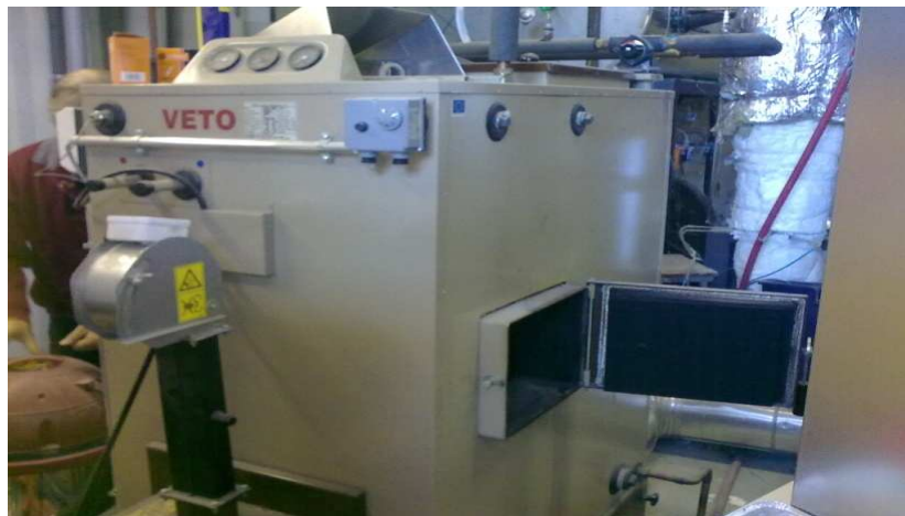
Picture 18. Front picture of VETO boiler at Energy laboratory of LUT /51/.
