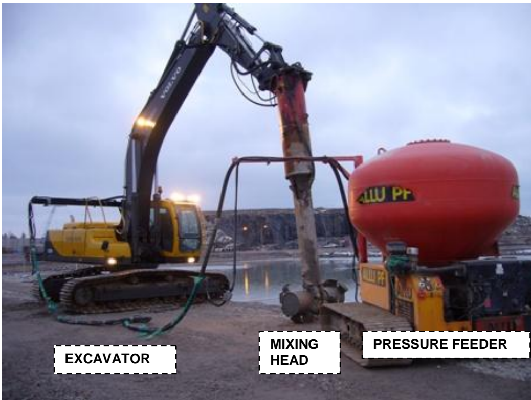
Figure 7.6. Mass stabilization machinery in Vuosaari (Helsinki) harbor contaminated sediment treatment project. Similar set up was used in Kokkola stabilisation project
