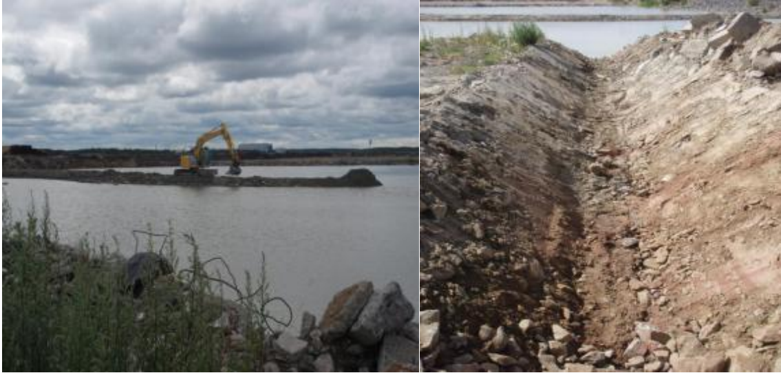
Figure 7.3 On the left is construction of the dumping pool, on the right is the constructed overflow ditch leading to overflow basin.
