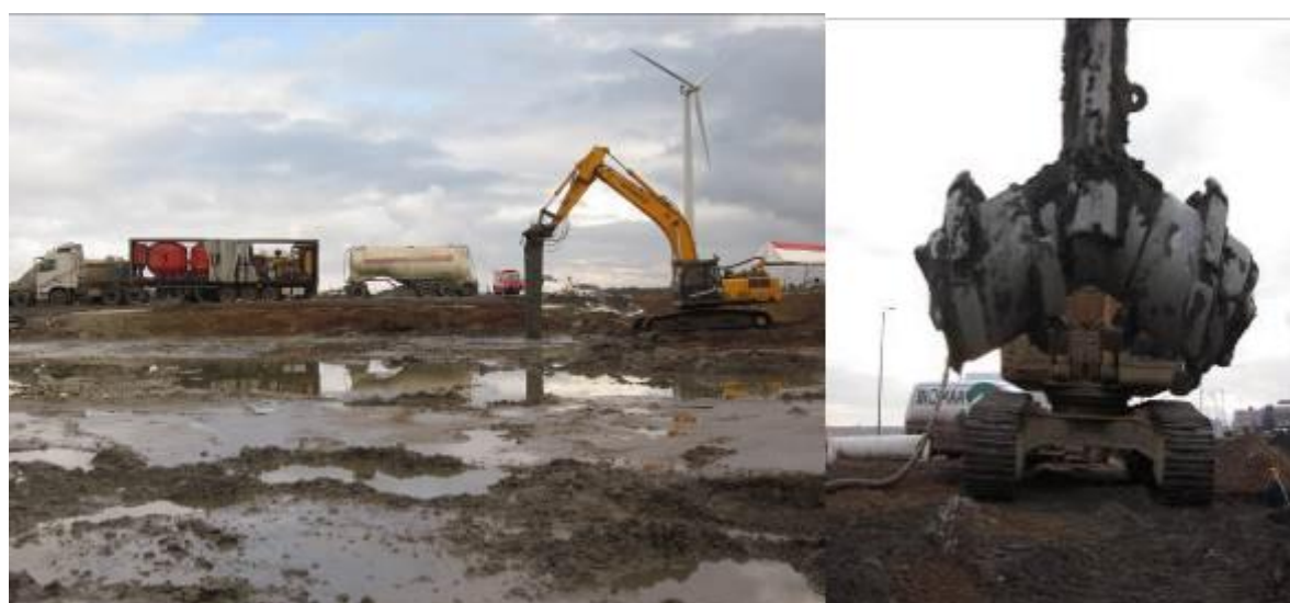
Figure 7.8. Mass stabilization equipment: binder storages and the feeding unit in left, the excavator with mixing tip and the outlet for binder materials in right.
