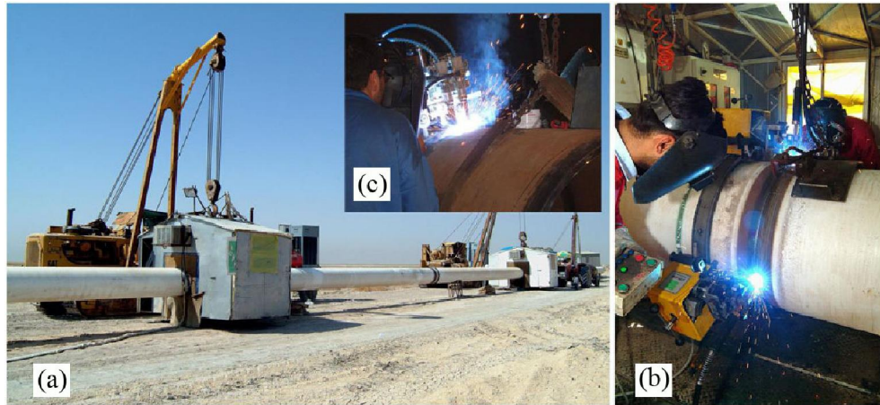
Figure 20 The pipeline and welding cabins (a), the welding robots inside the cabins (b and c) [129, 130]
