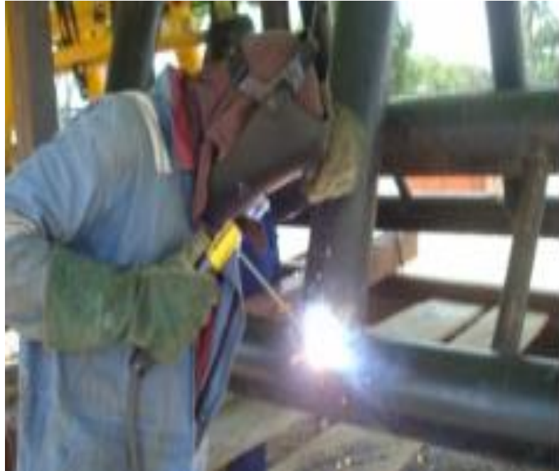
Figure 24. Welding of tubular offshore support structure with SMAW (courtesy of Seaweld Engineering).
