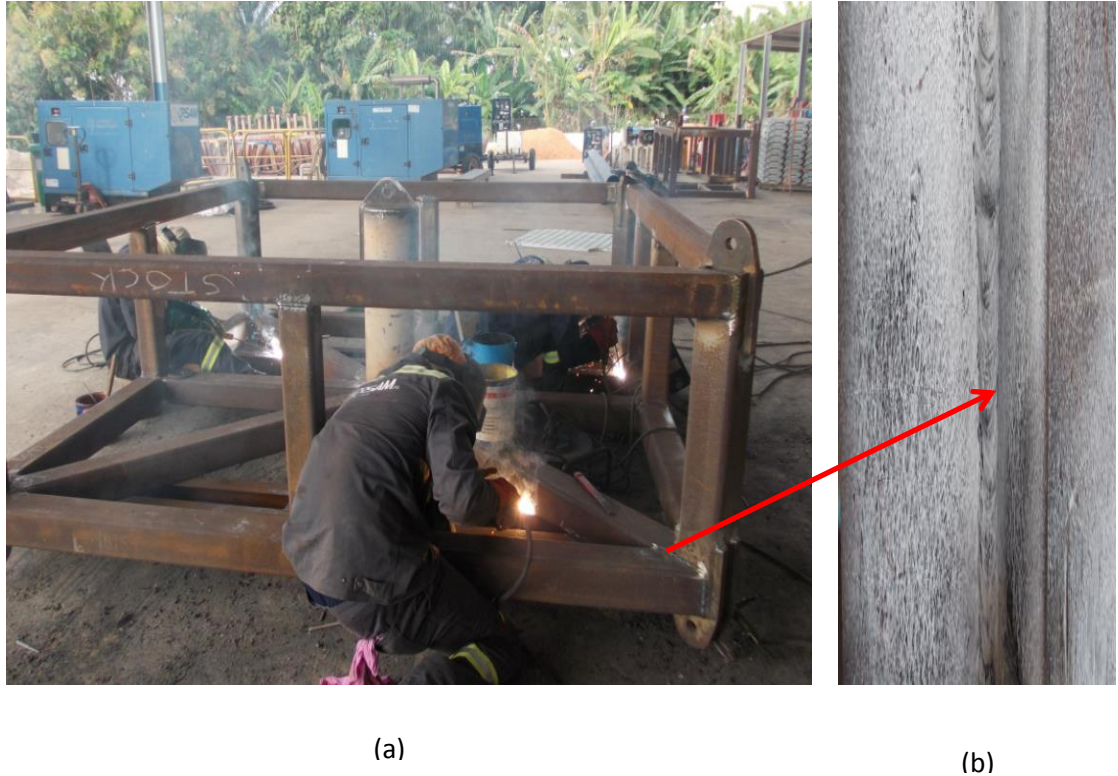
Figure 22. (a) Welding operation utilizing SMAW process on an offshore support structure. (b) Magnetic particle test of the welded joint of the offshore support structure.
