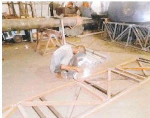
Figure 43. Manual welding of a steel grid structure in Socafer A.S, Cameroon (courtesy of Paul Kah, Lappeenranta University of Technology).
