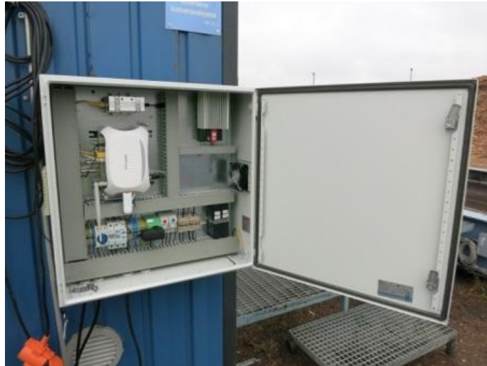
Figure 16 The reader unit was inside the cabinet.
