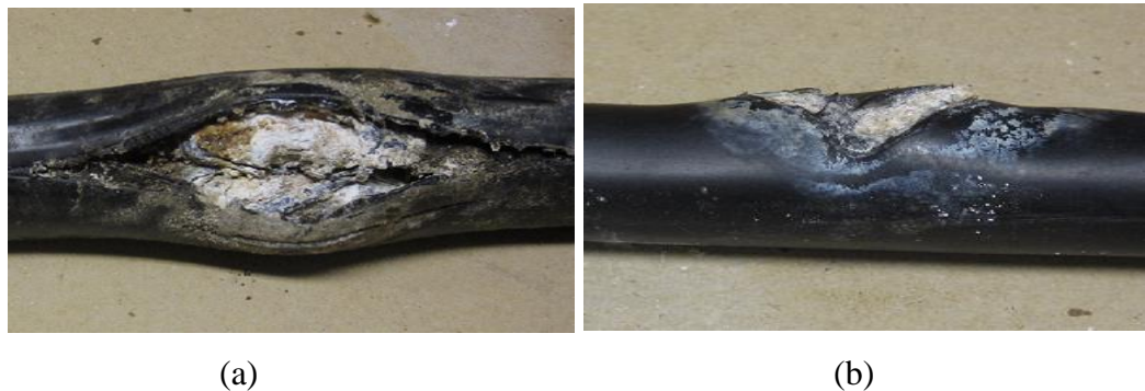
Figure 1.3. Damaged insulations. (a) Totally damaged insulation material of LV underground cable, caused by incorrect manipulation during the plugging process or installation, (b) insulation material damaged by a screw [15].
