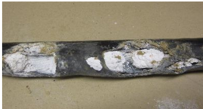
Figure 1.2. One phase, totally damaged LV underground cable, aluminium oxide broke the sheath [15].
