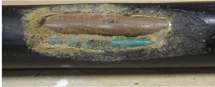
Figure 1.4. Power cable gnawed by a mole, but still working. Replaced to avoid a future fault. [15]
