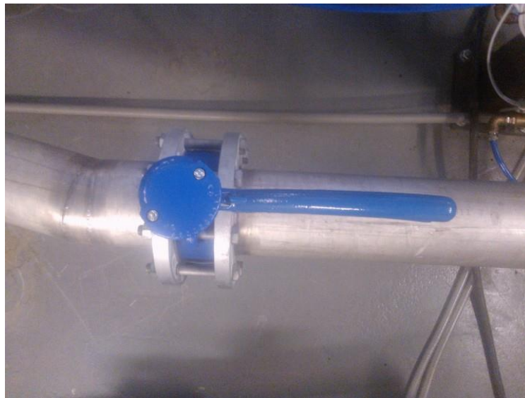
Figure 5.8 Manual throttling valve at the suction side of the pumping system. The valve had 10 possible positions ranging from fully open to completely closed valve. The amount of NPSH_a can be reduced by closing the valve.
