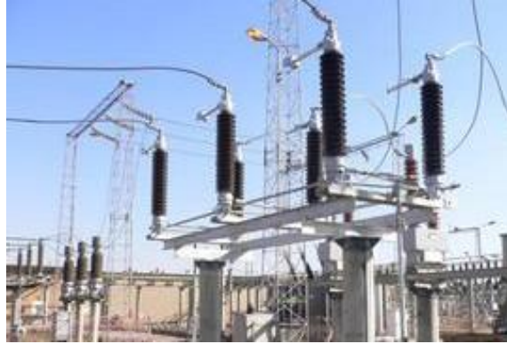
Figure 4.15. HV remote-controlled disconnector [9].
