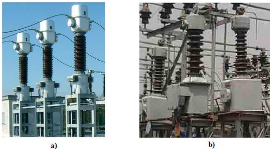
Figure 4.11. 110 kV instrumental transformers: a) – current transformer; b) – voltage transformer [9].
