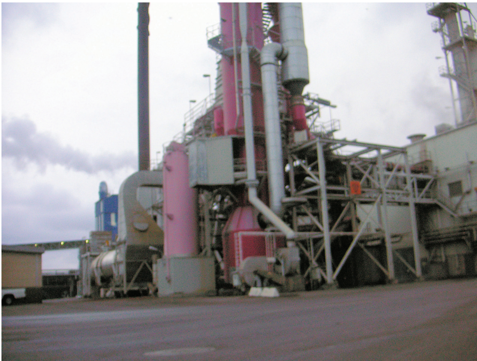
Figure 7. CFB gasifier connected to a lime kiln in Värö
