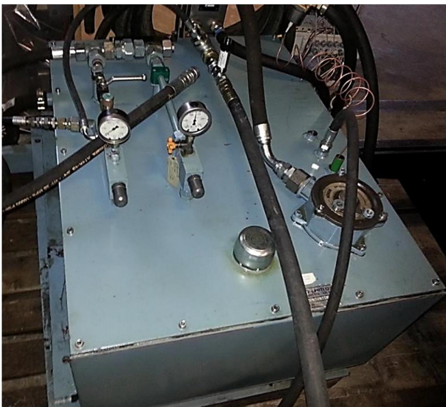
Fig. 10. Hydraulic oil tank.
