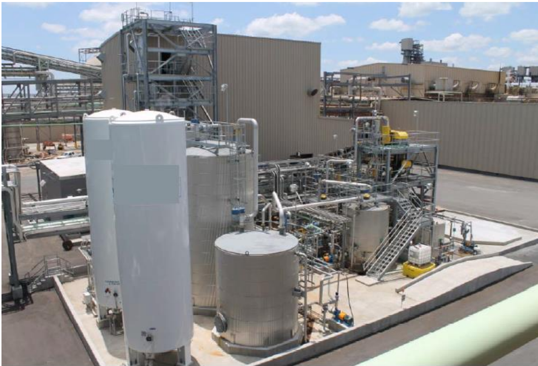
Figure 5: An industrial lignin separation plant at Domtar, Plymouth (Tomani 2013).
