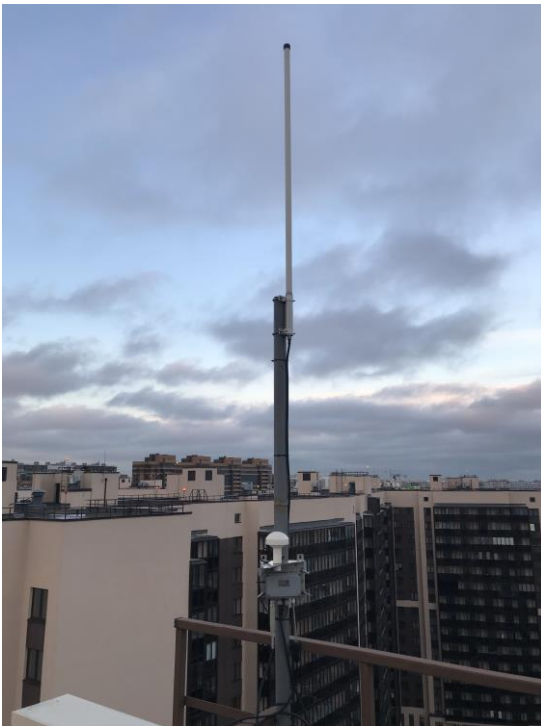
Figure 34. LoRaWAN gateway with antenna 10 dBi (Murino district, Saint Petersburg).
