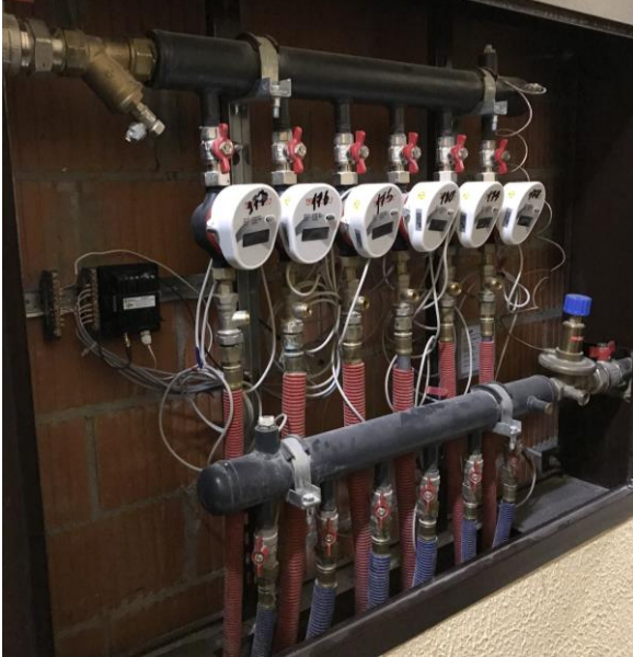
Figure 33. Heat meters with M-Bus interface equipped with M-Bus-to-LoRaWAN converter (Murino district, Saint Petersburg).
