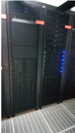
Cold aisle containment
