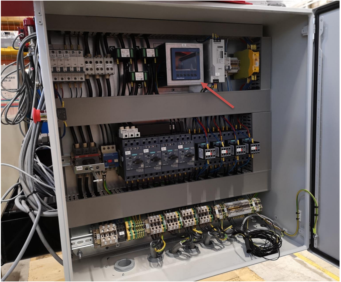
Figure 29. Location of the energy measurement device (shown with an arrow) in the power supply cabinet.
