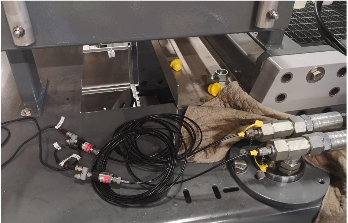
Figure 26. Pressure transmitters fitted in the ports of cylinder four.
