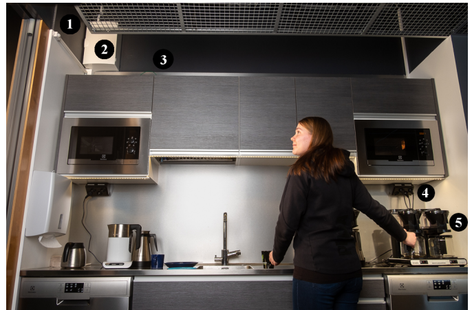
Fig. 1. Break room where the platform is located. Daily activities are not affected by the sensor placements: IR sensor (1) monitors movement. Brewing of coffee is monitored with a multifunction power analyzer located in the breaker panel (2). The analyzer measures the energy consumption at the electrical outlets (4) that power the coffee maker (5). Environmental data are measured with a Bluetooth beacon located next to the Raspberry Pi (3), into which all data are collected. Raspberry Pi also acts as an IoT controller and a gateway to the Internet.
