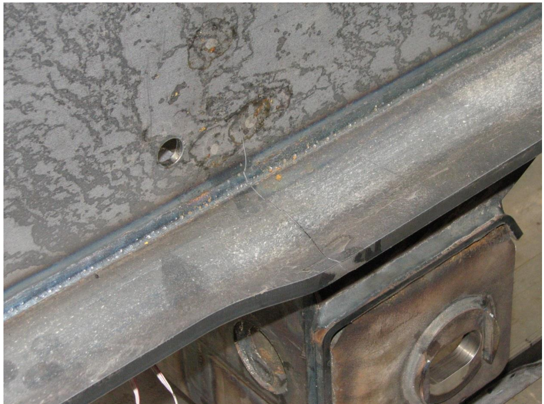
Figure 40. Weld toe crack.
