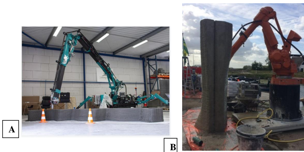
Figure 8A. Off-site 3D printing by robotic arm ( Constructions-3D MAXI PRINTER review - mobile construction 3D printer ,). B. on site printing by robotic arm ( 3D concrete printers / CyBe Construction ,).
