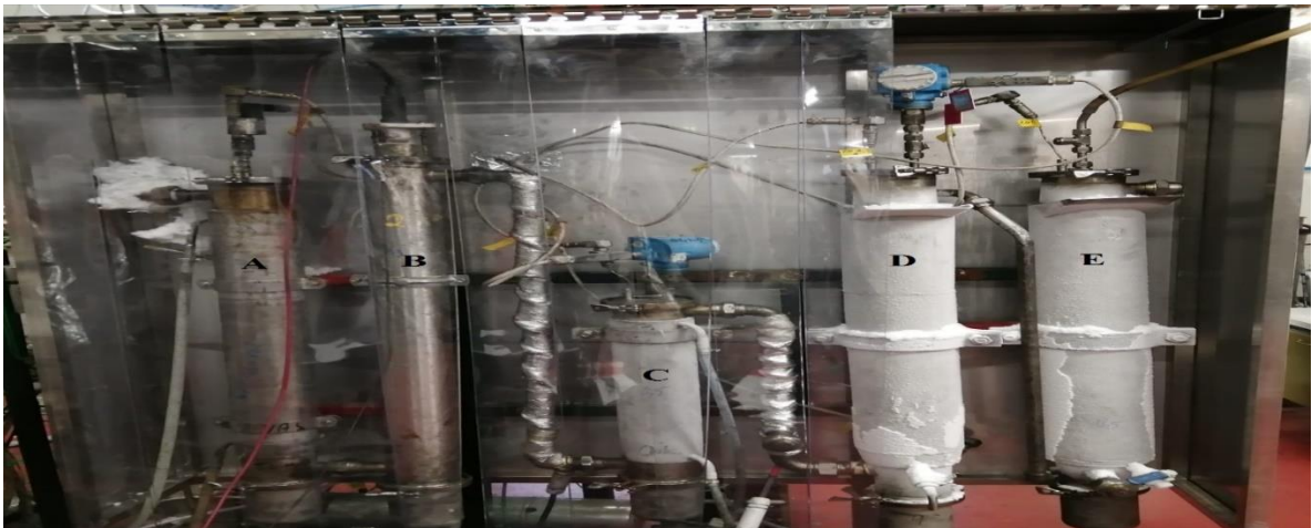
Figure 16: Cooling Section of Kilo reactor
