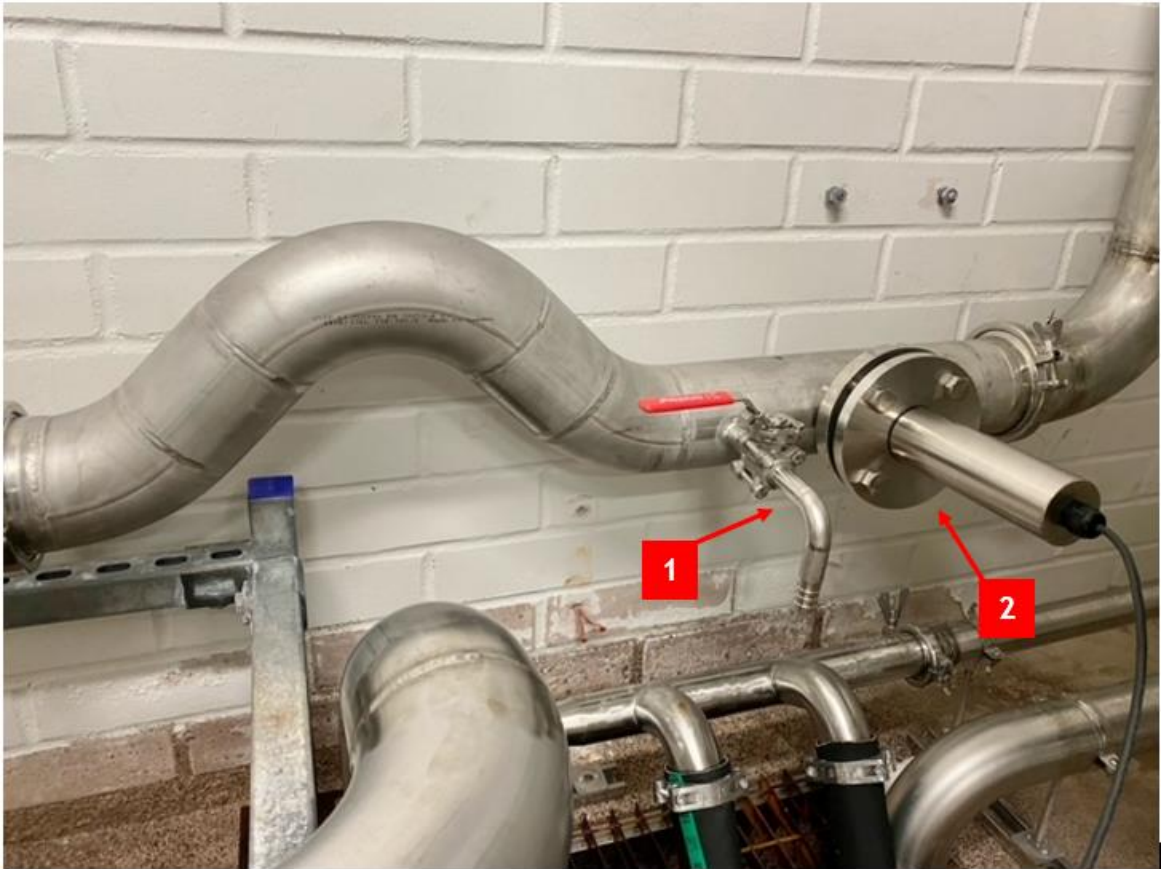
Figure 11 Sampling valve (1) and Collo Plate analyzer (2) in the pipeline.
