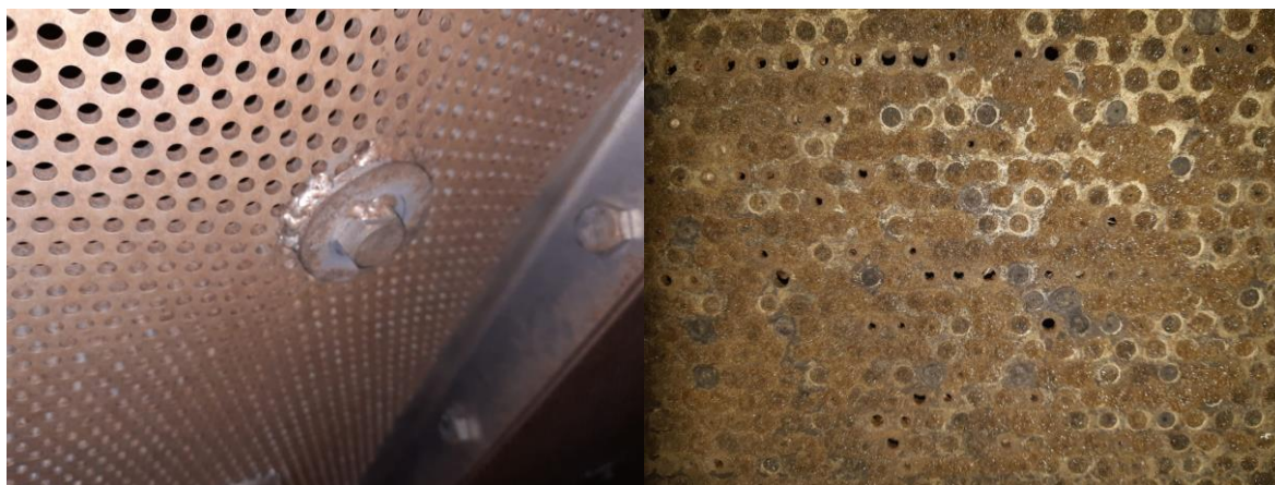
Figure 6. Scaling can also gather up mass from cooking over time, plugging the screen.
