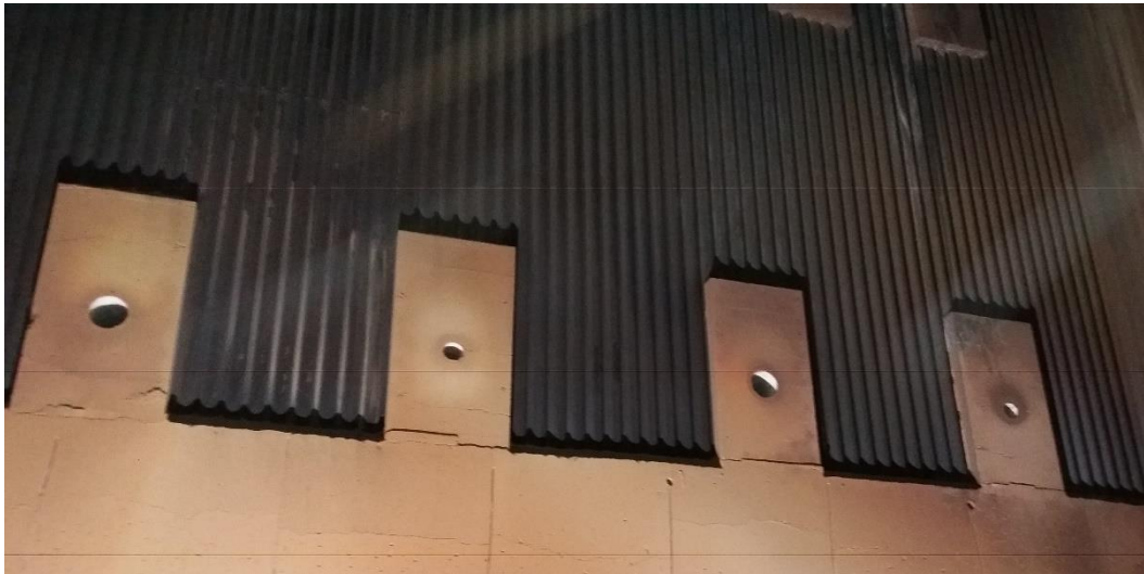
Figure 5. Lower secondary air nozzles of a new and clean BFB boiler (SHI FW internal material, 2022).
