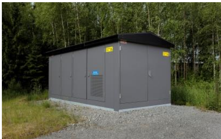
Figure 7. Transformer cabin example (Alfa Elkamo, 2023)
