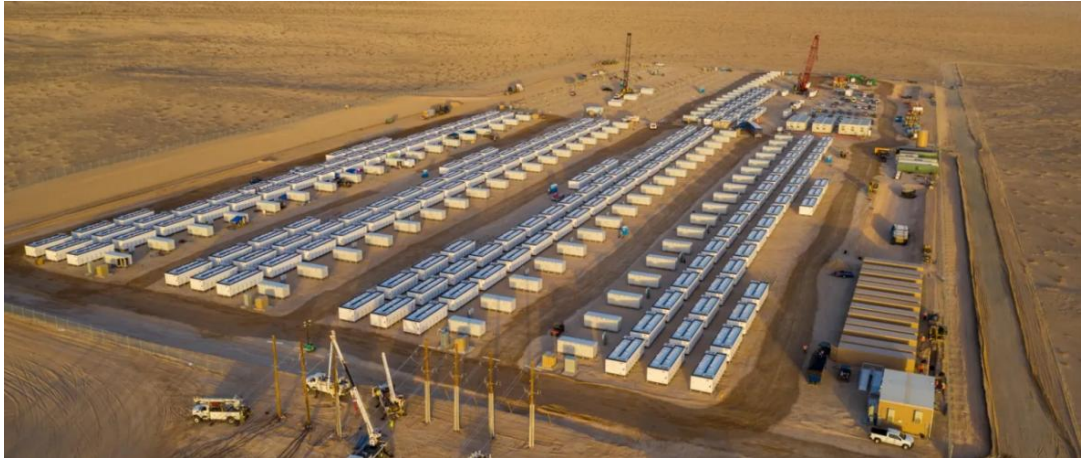
Figure 20. The world's largest battery energy storage system adopted from [52].
