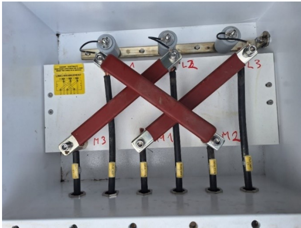
Figure 5.2. Picture of a bonding lead link box internals.
